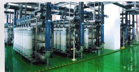
Waste Water Re-use | 1000m³/h
