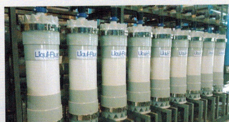
Process Water Power Plant | 240m³/h
