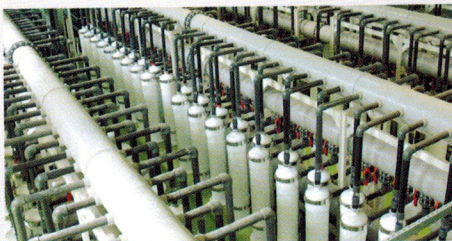
Waste Water Re-use | 2250m³/h
