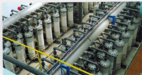
Pre-treatment to Reverse Osmosis | 540m³/h
