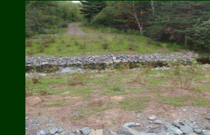
Culverts are removed, the stream bed restored and banks replanted to improve fish habitat.
