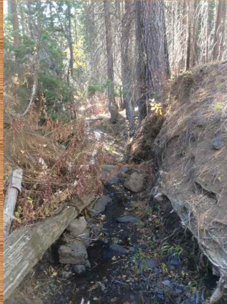
Old log culvert in upper Boulder Creek with oversteepened banks on road proposed for storm damage risk reduction treatment (lay back and stabilize banks until next entry).
