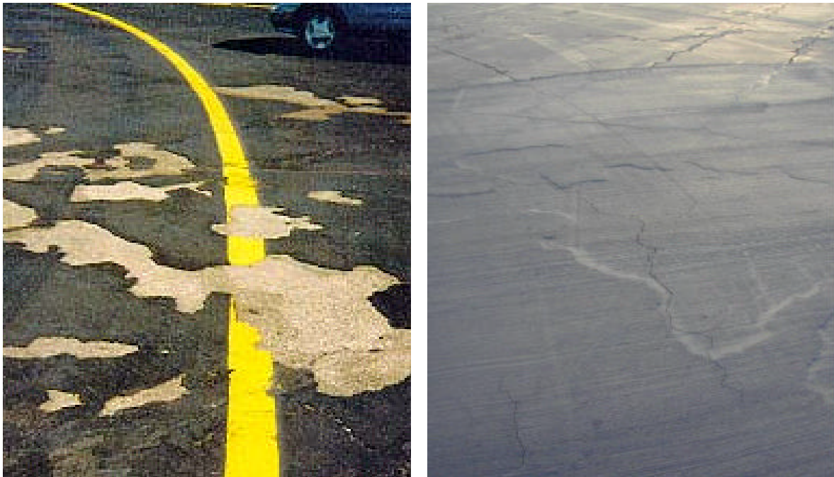
Figure 7. “Delaminated coal tar area before (2008) and after sealing with PCMO (2012) at Forbes Field, Topeka, KS.
