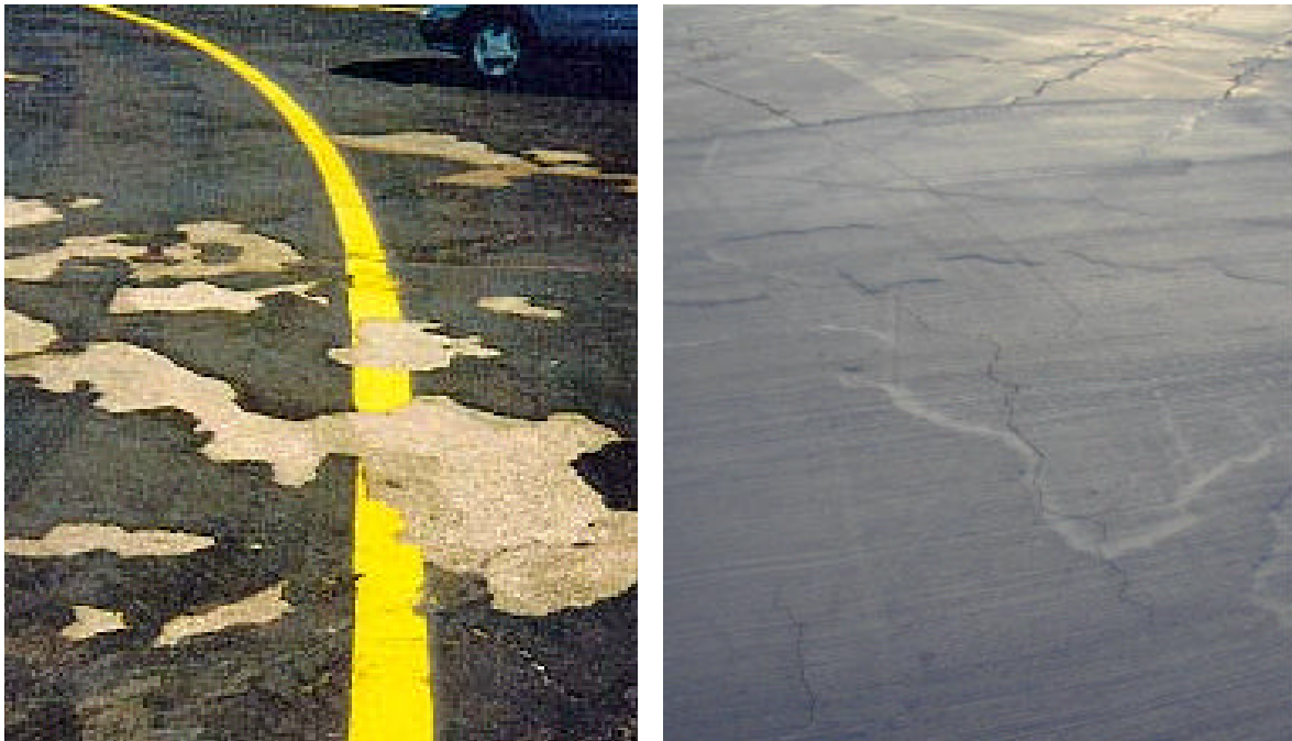
Figure 7. “Delaminated coal tar area before (2008) and after sealing with PCMO (2012) at Forbes Field, Topeka, KS.
