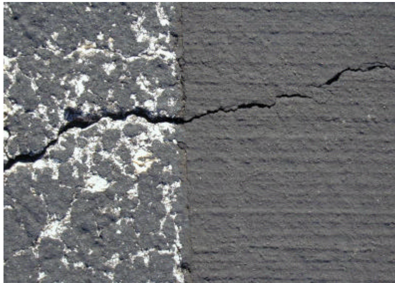
Figure 5. PCMO section at MacDill AFB showing reflective cracking. Note that the crack has not widened or displayed any raveling from the crack face.
