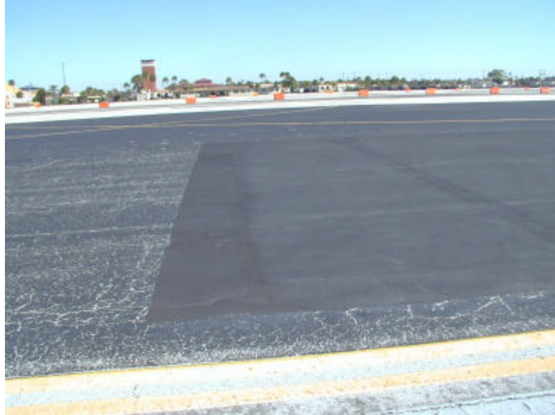
Figure 4. PCMO surface in October 2012 at MacDill AFB. The adjacent pavement is coal tar that is approximately 14 years old and is severely deteriorated.
