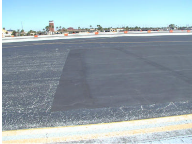
Figure 4. PCMO surface in October 2012 at MacDill AFB. The adjacent pavement is coal tar that is approximately 14 years old and is severely deteriorated.
