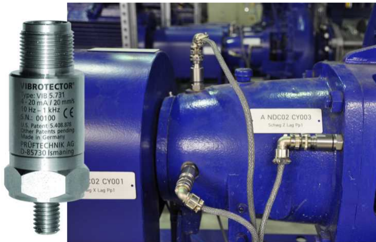
Monitoring vibrations with VIBROTECTOR
