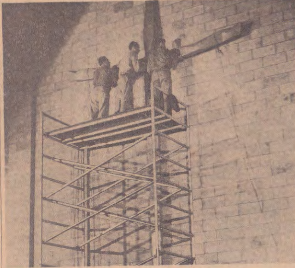
The crosspiece of the cross in the new St. Luke's Episcopal Church is put in place in preparation for the first service in the Haworth church on Easter Sunday. Putting the crosspiece in place are Charles Walden, Edgar Anderson, and Donald Edson. Anderson and his
